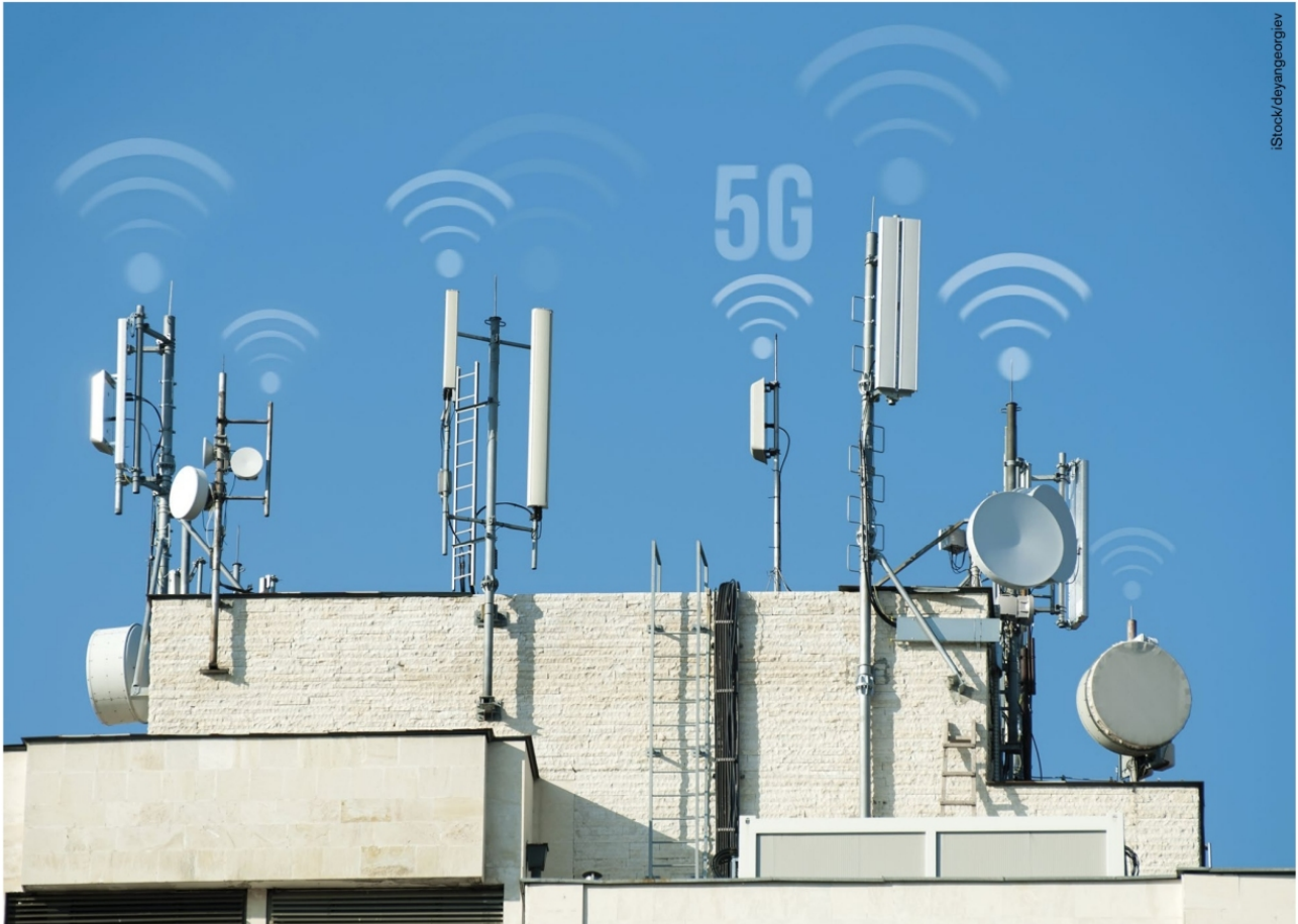
The FCC is authorizing the deployment of hundreds of thousands of small cells with little public input or environmental review.
