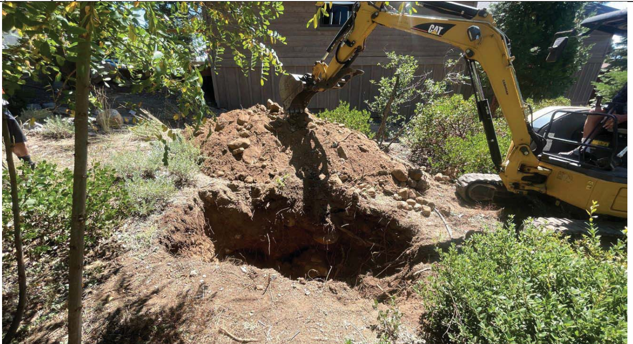
Photo 4 – View to southeast edge of parcel where Test Pit no. 1 was excavated by backhoe. The pit was located about 35 feet west of Observation Drive and 15 feet north of the south property line. Slopes are 15% in this vicinity. The test pit showed the property has deep soils that become increasingly more gravelly with depth (no root restriction nor evidence of seasonal water table).
