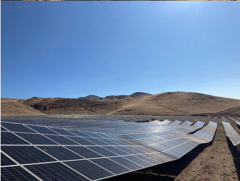
Example of solar array using ground screws and natural contours
