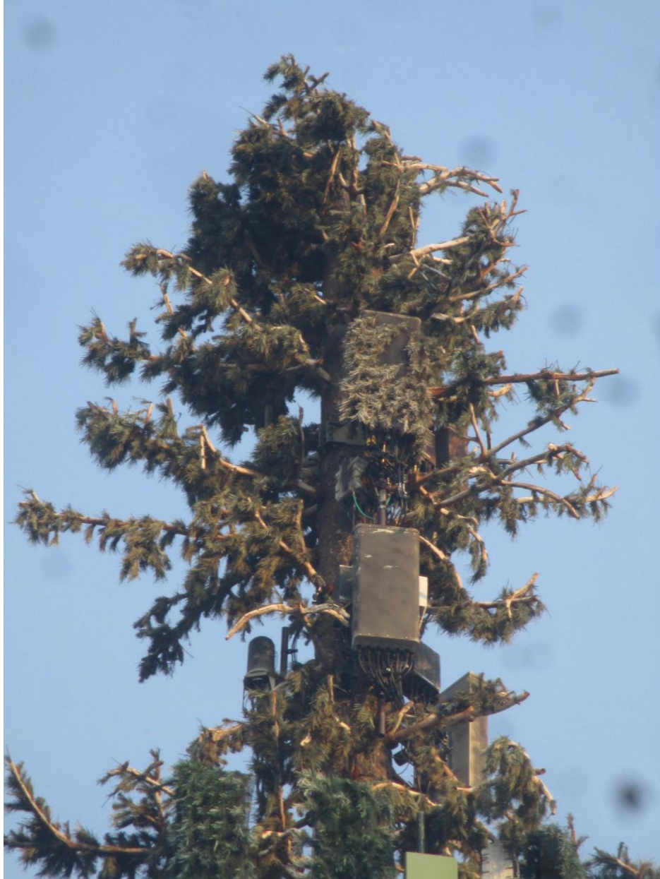
Closer view of Wilson Ave Tower. Note limbs missing needles, antennas lacking (required) covers.
