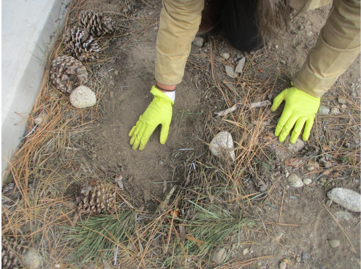
Needles discarded at base of Keetak Drive macrotower prior to onset of fall snow cover, not isolated, but representative of the clumps and needles dispersed around the tower debris field.
