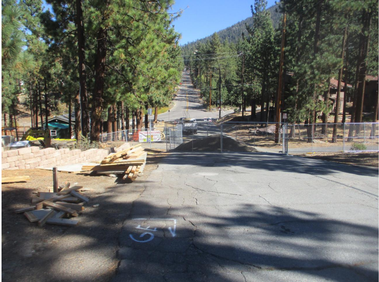
Verizon committed to keep all the soil on the Project site at the September 2022 TRPA appeal hearing for expanded foundation excavation. Soil is piled in Needle Peak Drive, Ski Run Blvd below to left. Street closed to public.
