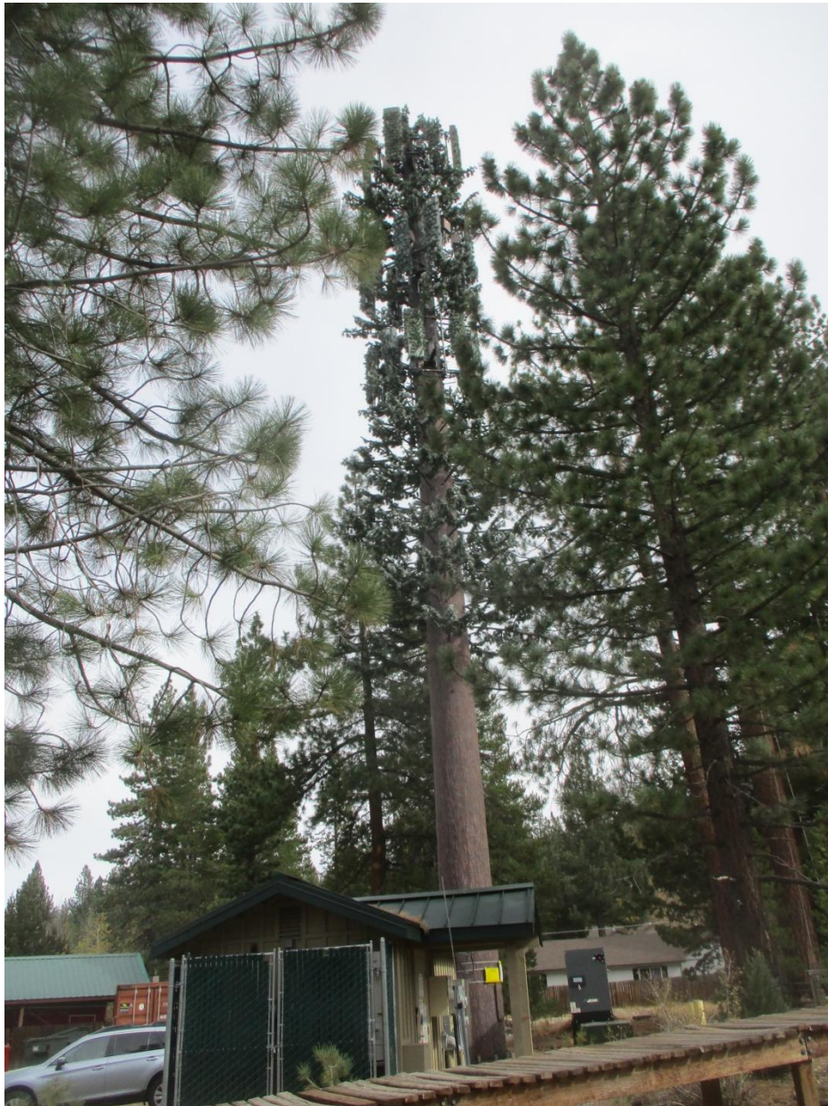
Tower base station viewed from near Hwy 89 entrance. Needles and plastic antenna covers on the tower appear to be degrading in situ and detach in wind and weather.
