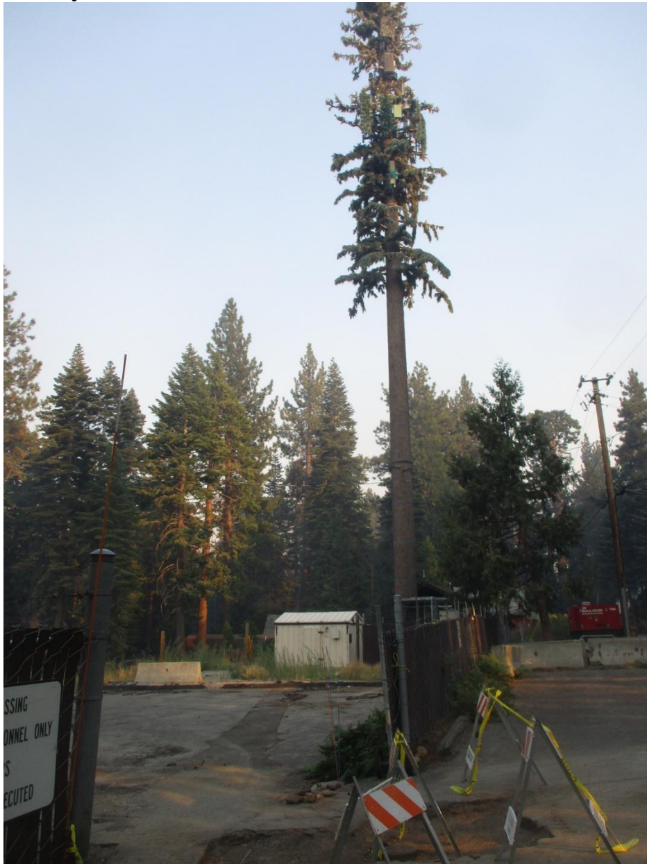
Wilson St. Tower from near entrance to El Dorado County maintenance facility (to left), looking southerly, Wilson Street/right of way at right of the fence. Note hanging broken limbs on tower and plastic coverings missing from antennae.
