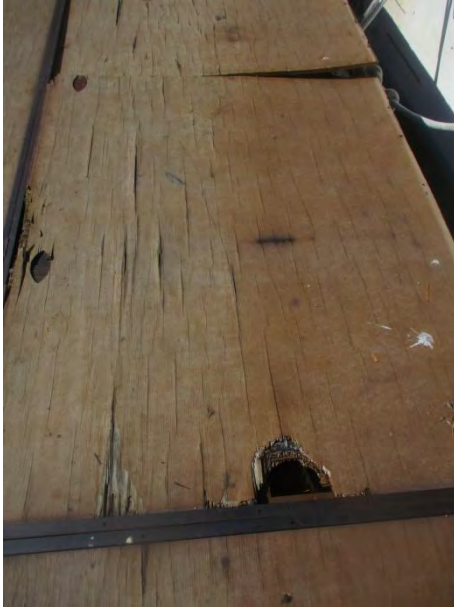
Deteriorating weathered plywood. (7993)
