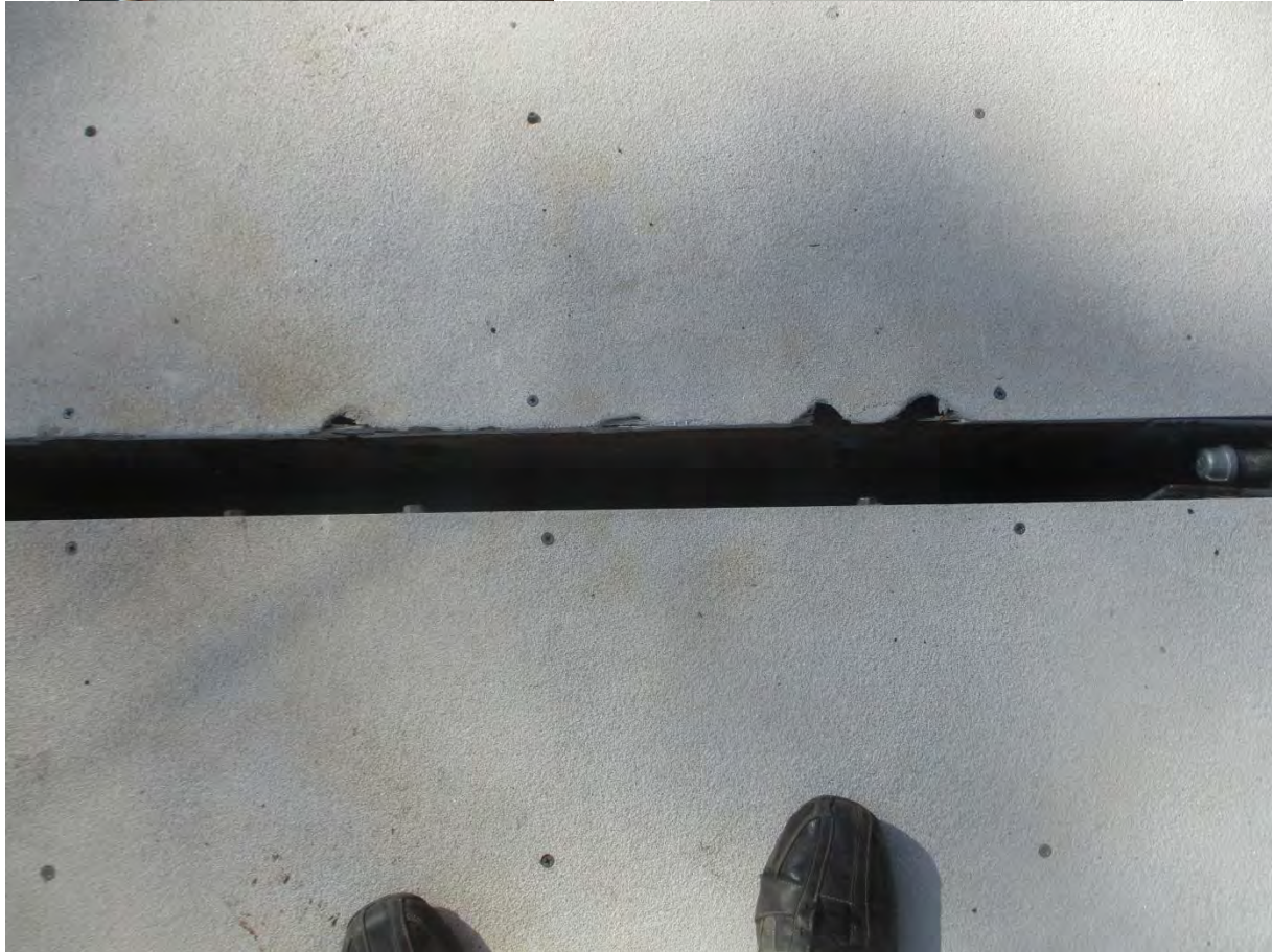
Fuel dock area, plywood and plastic panels. Note cracking, abrasions. (8020) (8022) (8023)
