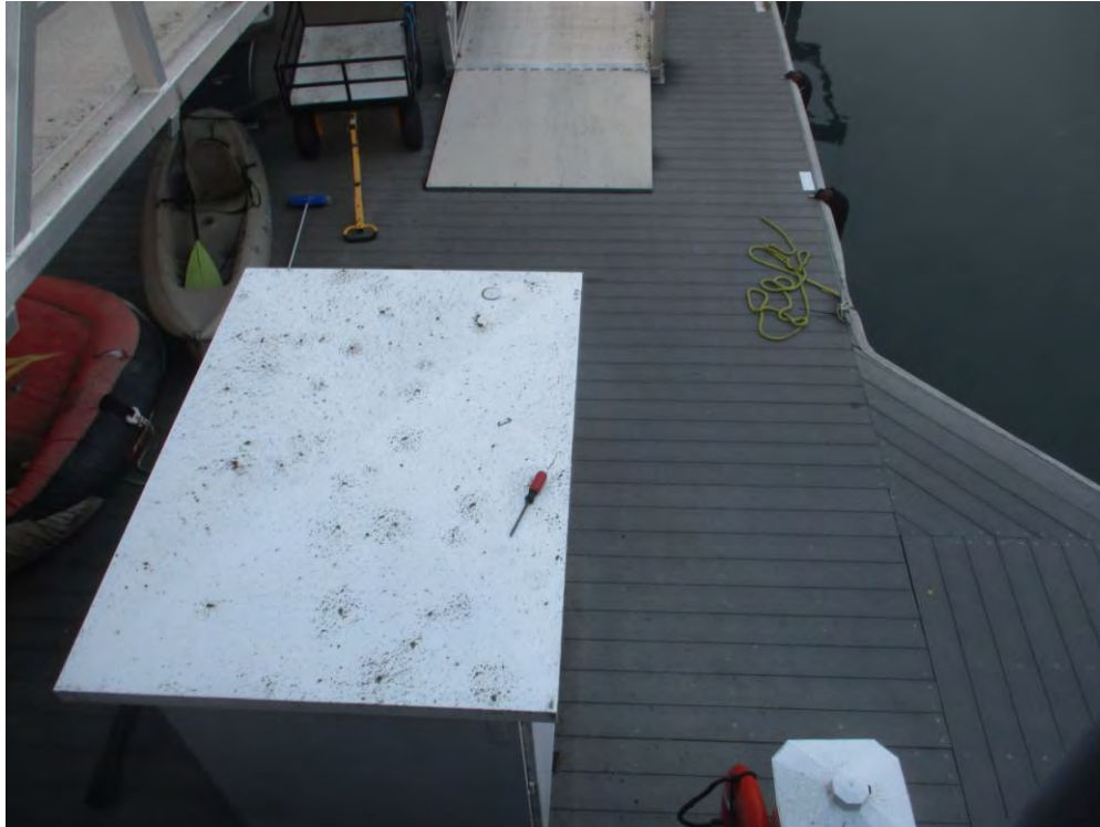
Example of decking in the older sections, ramp at top of photo. (5464)
