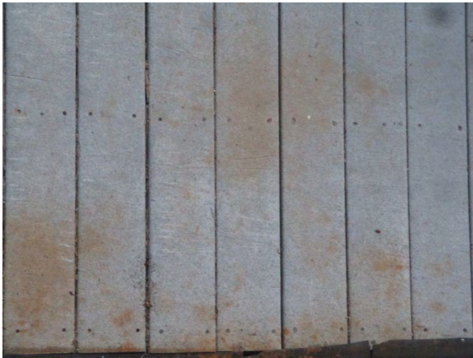
Weathered, scuffed, scratched, stained decking. (5485)
