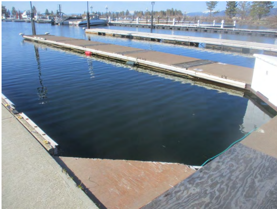
Some older pier decks are concrete, which hold up better, or wood. Here is a floating dock extension (above center pier, whitish) that is partly covered by plastic sheathing. (8011)
