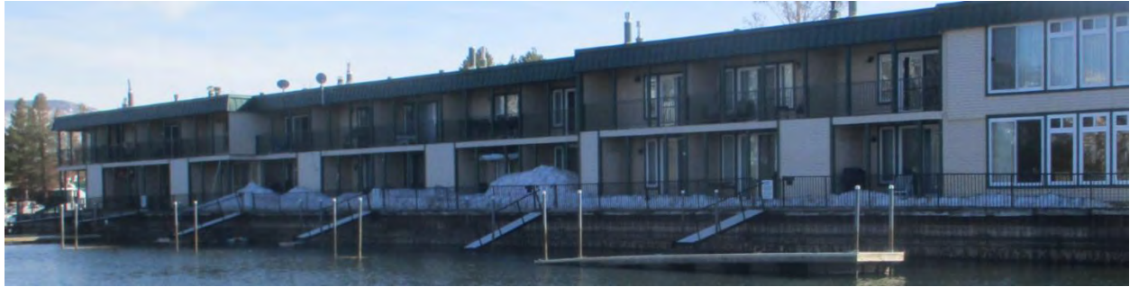
Four of six boat ramps missing docks, broken and submerged by winter snow and ice, post-thaw. Condo side, facing southerly. (7985)
