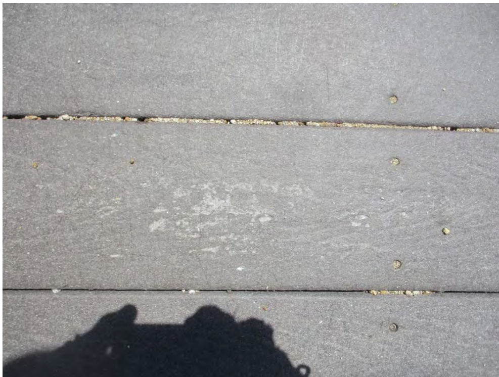
Close up of typical plastic decking showing weathering, surface wear and scratches from sand. (4245)
