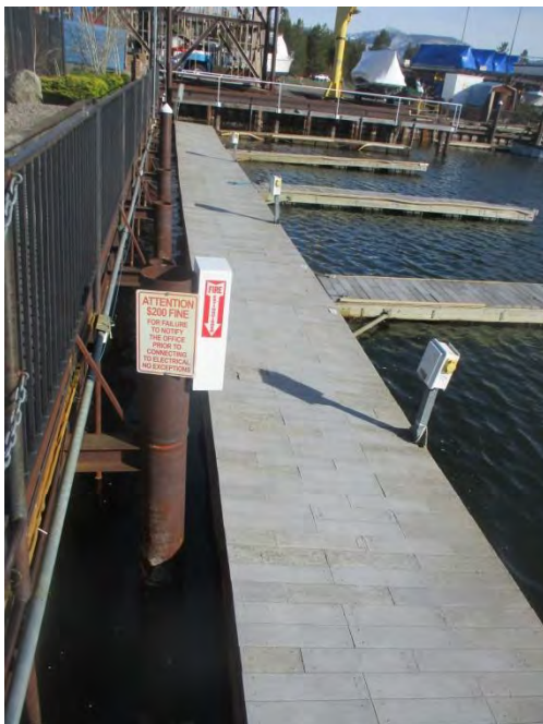
Deteriorating “checkerboard” decks, south end with boat hoist shown, top middle. Popcorn in water. (8062)
