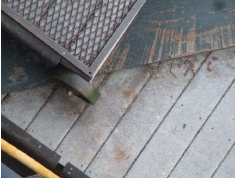
Abrasion at ramp connections, weathered plywood. (5484)
