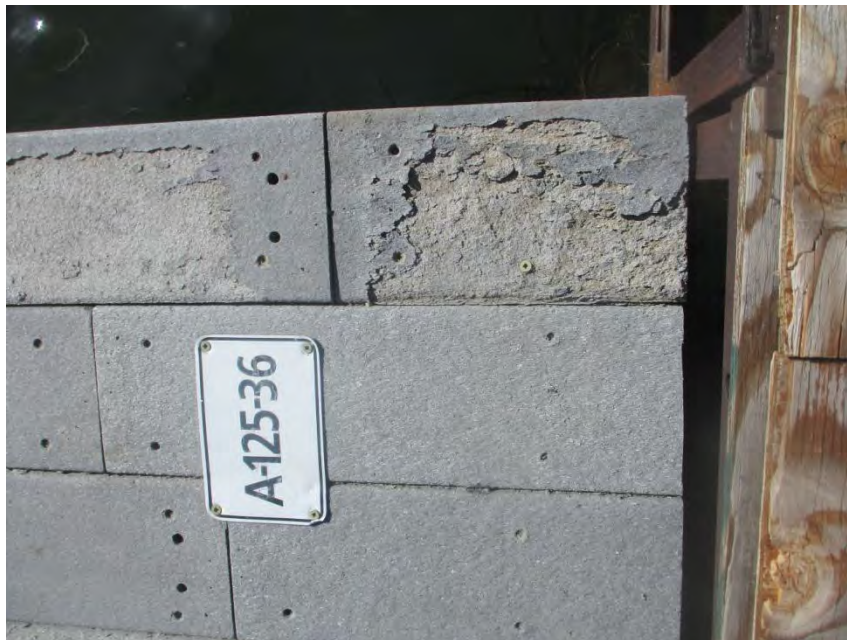
Plastic decking deteriorated from weathering and flaking off as microplastics over waters. Typical of the hundred of plastics docks at Tahoe Keys Marina. (7982)
