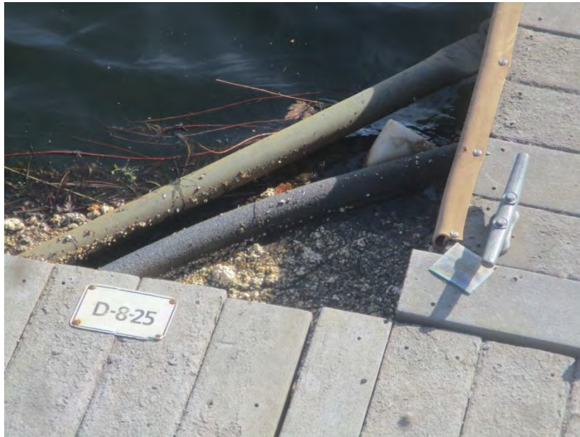
Deteriorating PVC decking, with polystyrene (PS) “popcorn” in the water from disintegrating ballasts. Tahoe Keys Marina. (8063)
