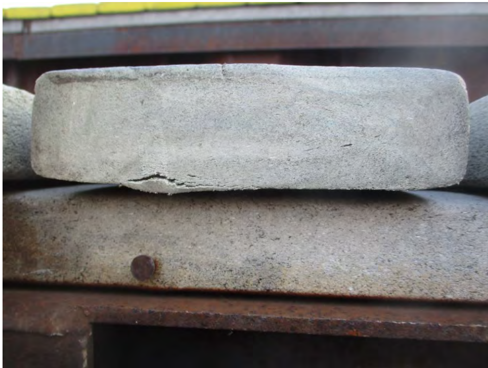
End-view of plastic deck boards showing cracking. (5430)
