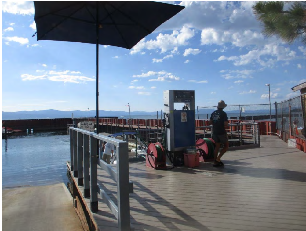
Small marina. Wrap-around plastic decking, generally in good condition, adjacent boat ramp. (50 31)
