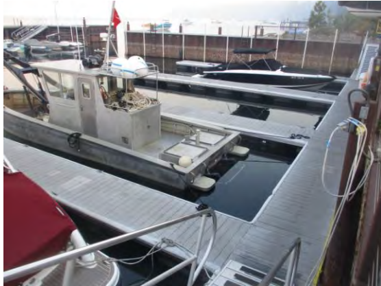
Checkerboard decks, ramp abrasion.(5410)
