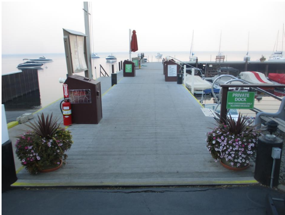
Looking easterly, fuel dock on far end. Note severely degraded plastic decking at entryway. All of the observed decking is in a state of decay at this marina, while still capable of serving functionally. Observations at Obexer’s marina include a high number of degraded deck boards, plastic with breakage, cuts, chips, abrasion and general deterioration, as follows. (5454)
