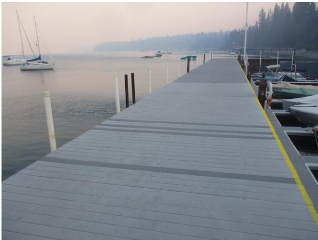
Some replacements were obviously needed. The material in the foreground is weathered, friable and subject to further weathering and dispersal. How bad did it get prior to replacement? (5438)
