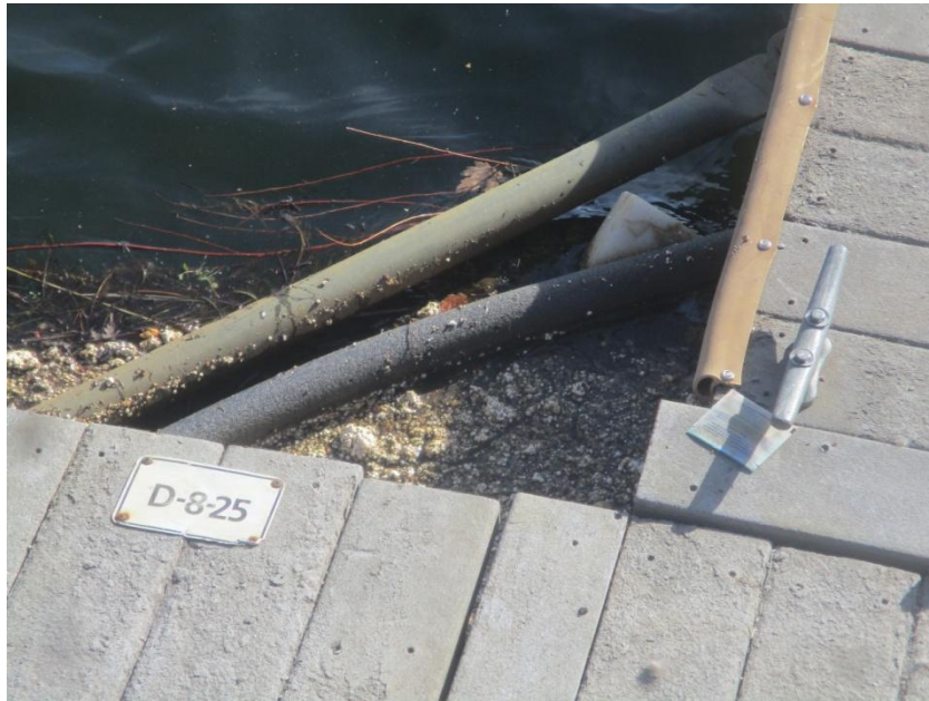
Deteriorating PVC decking, with polystyrene (PS) “popcorn” in the water from disintegrating ballasts. Tahoe Keys Marina. (8063)
