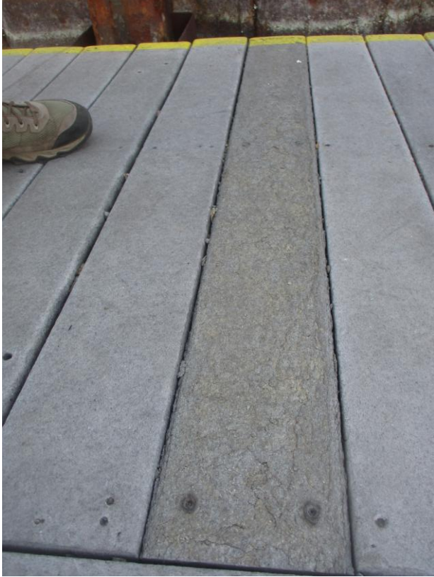
Severely weathered plastic deck board with other less-weathered plastic deck boards.(5420)
