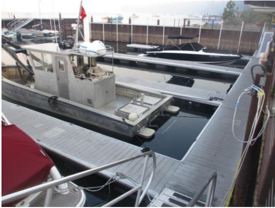
Checkerboard decks, ramp abrasion.(5410)
