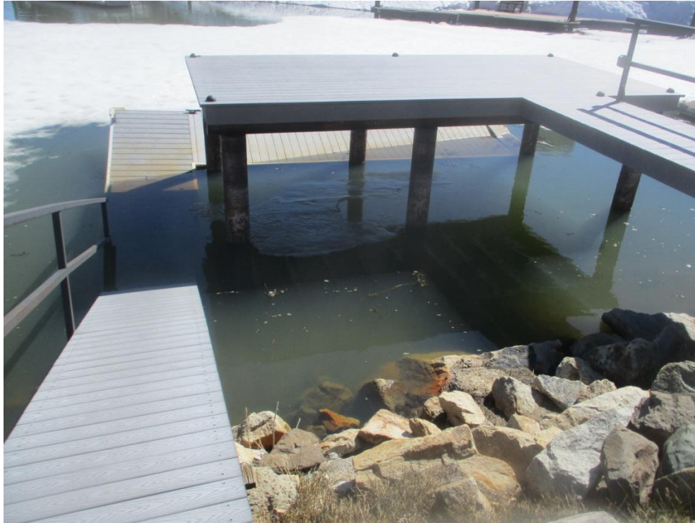
Submerged plastic dock, typical of the many that will require repairs following the winter of 2022-2023. (7513)
