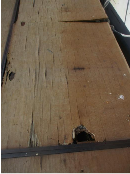
Deteriorating weathered plywood. (7993)
