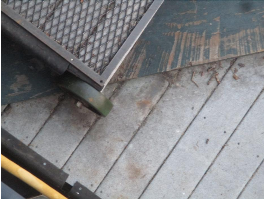
Abrasion at ramp connections, weathered plywood. (5484)
