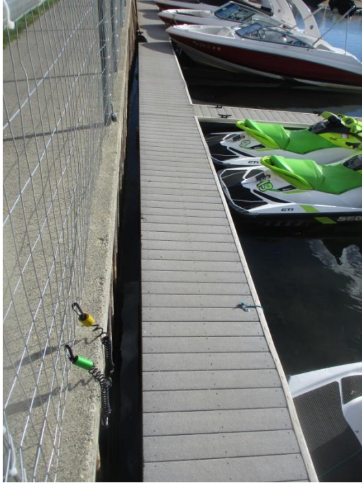
Some minor weathering and surface deterioration of decking on close inspection. (5033)
