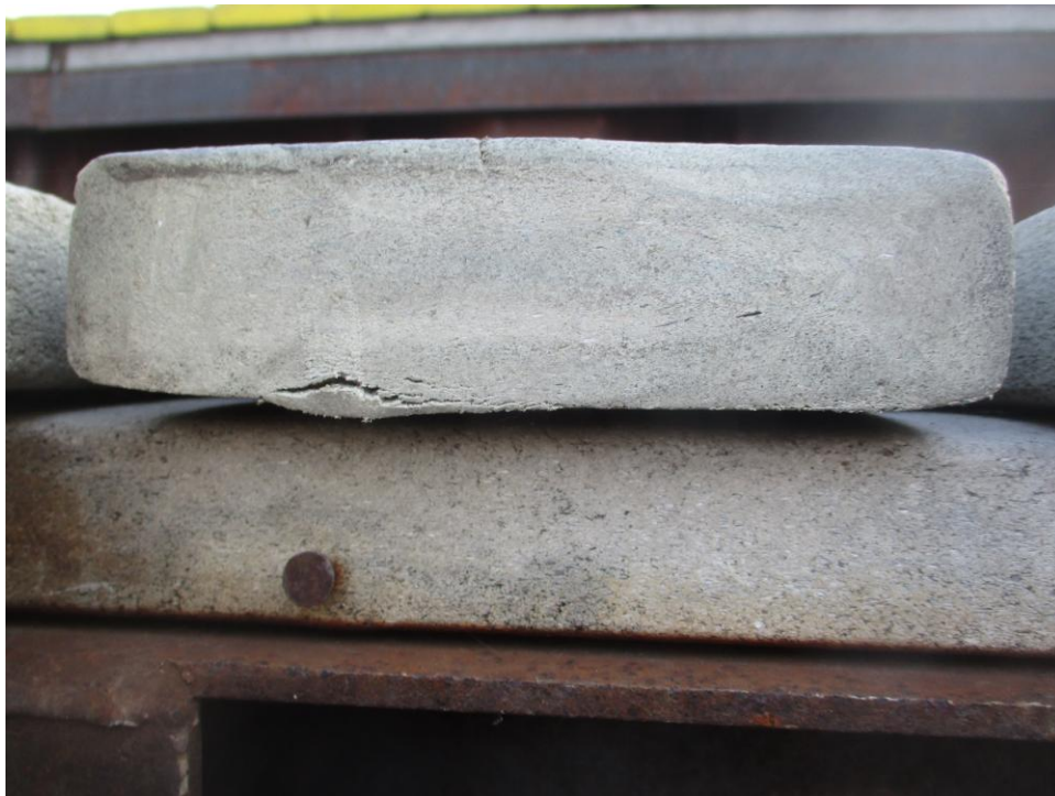
End-view of plastic deck boards showing cracking. (5430)
