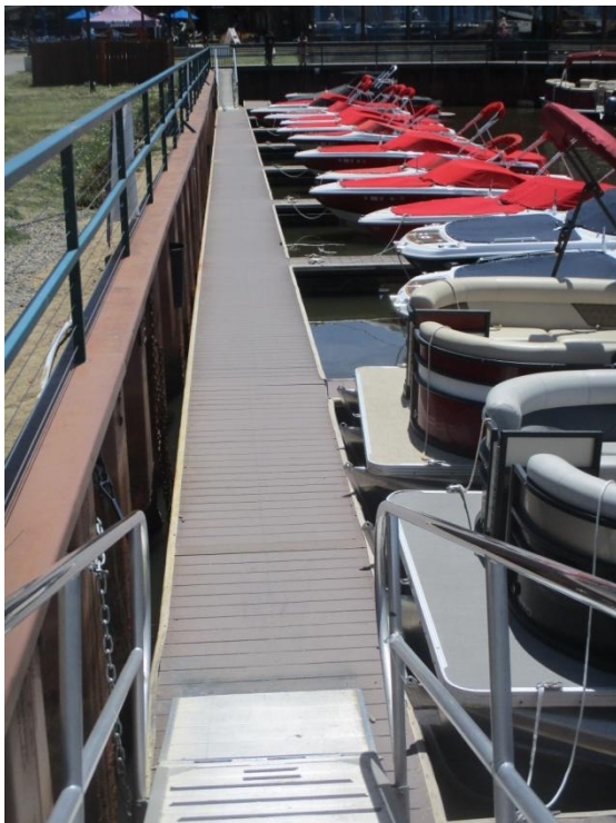
Abrasion of plastics at metal ramp interfaces is typical. (4231)
