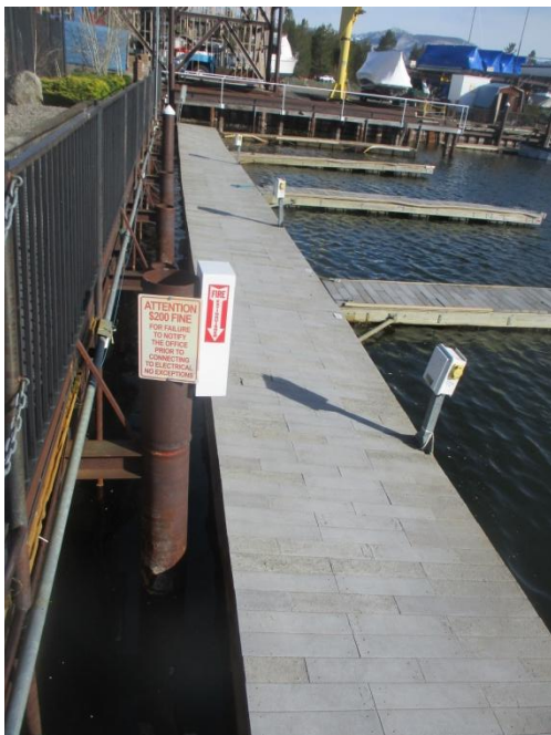
Deteriorating “checkerboard” decks, south end with boat hoist shown, top middle. Popcorn in water. (8062)
