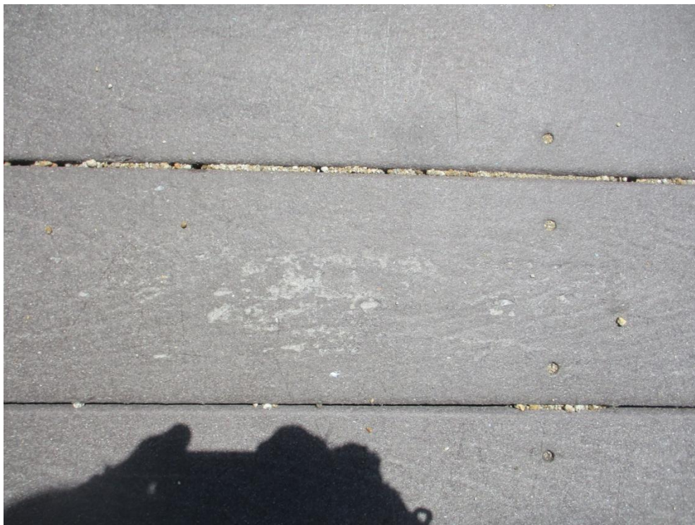
Close up of typical plastic decking showing weathering, surface wear and scratches from sand. (4245)
