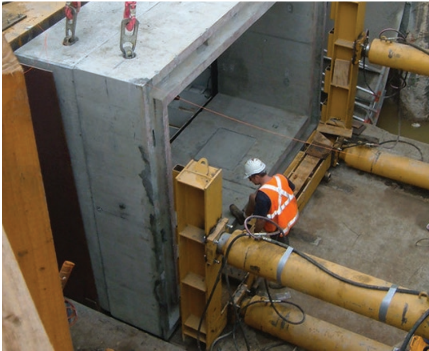
Figure 4.29: Culvert jacking may be an option for undercrossing construction (photo by tunnelcorp.com/au)
