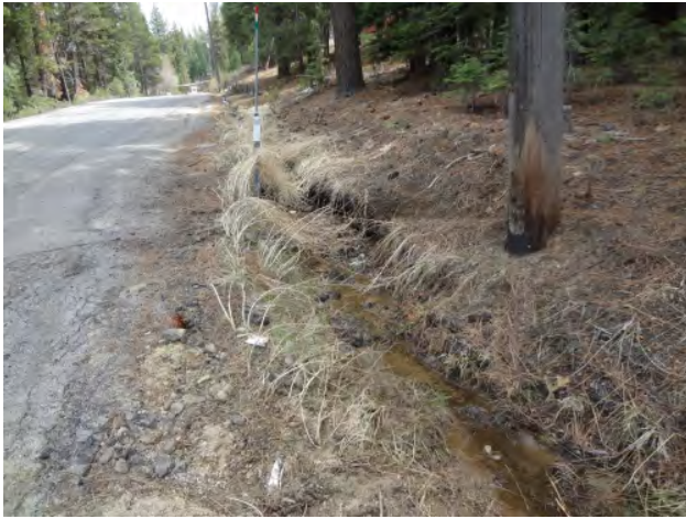
Phase 1/2 - Eroding channel
