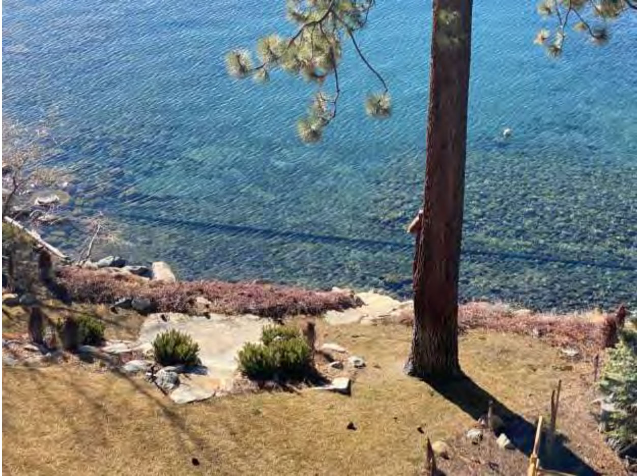
Exposed Sewer Pipe 1/20/2020
