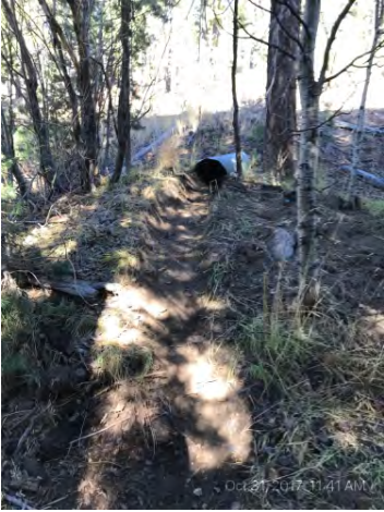
Outfall at Pioneer Trail - drains Crystal Air and Oflyng
