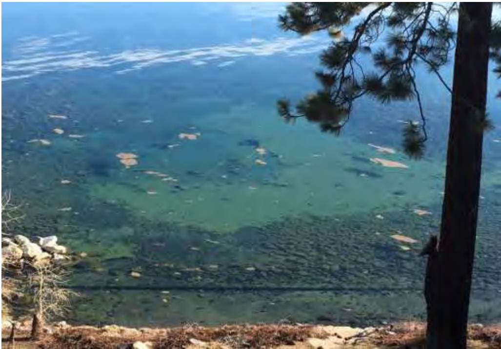
Exposed Replacement Pipe Photographed on 3/31/2019 – Twelve Days After Completion
