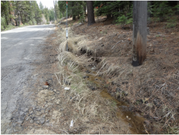
Phase 1/2 - Eroding channel
